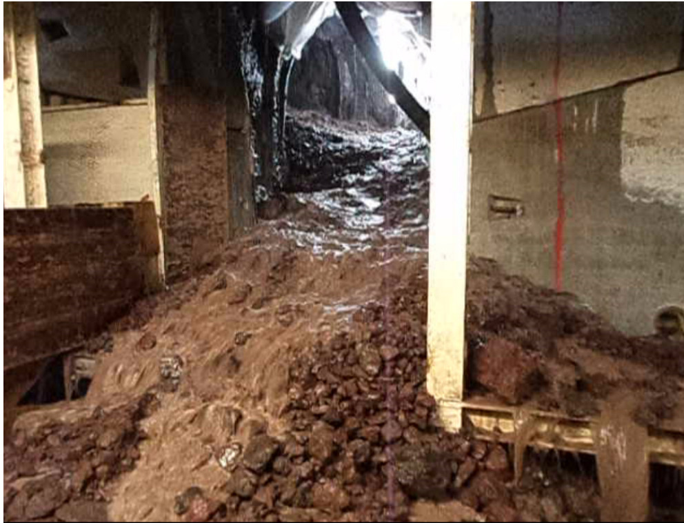
Figure 2. Of the three standard Double Shield TBMs used to originally bore sections of the tunnel, two became irretrievable stuck or damaged amid massive mud and water inflows.
