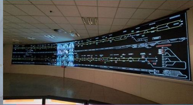
5. Athens Metro Lines 2 & 3: Operations Control Centre
