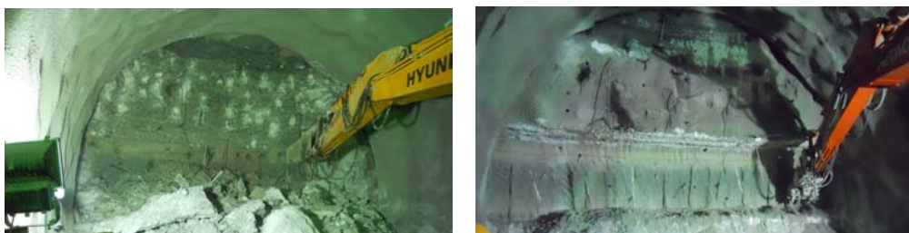
Figure 5. Mudstone and gypsum strata present on the WS5 at the TBM depth
